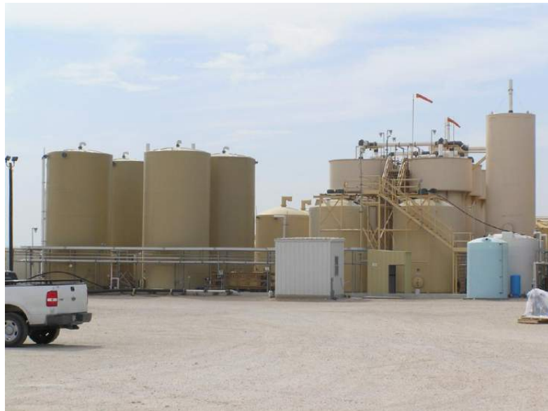
Figure 26 – The MULLC Processing Plant. (Additional Views of the Plant are Presented in Appendix II)
