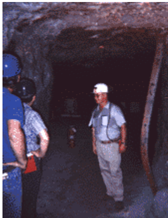
Photo 1: A door frame was significantly warped from salt movement over the last ten years.
