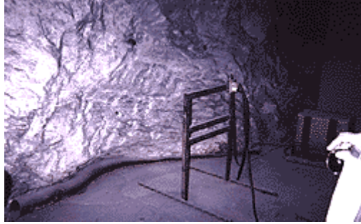
Photo 2: A pipe lying on the floor had been overridden by salt flow.
