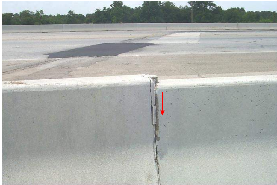
Figure 63 – Recent Movement in Retaining Wall at North End of Willow Creek Bridge New Repair Shown in Road at Bridge Edge. Looking East Across Highway 249.
