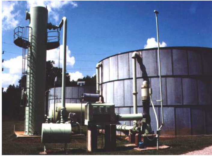
Figure 30 – MUD Well and Storage Facility at FM 1960 w/ De-Gassing & De-Sanding Equipment (From Campbell and Wise, 2013)
