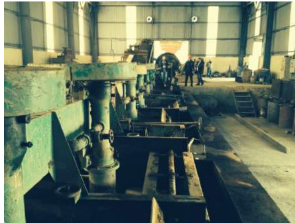
Figure 66 – Flotation Cells at the Processing Plant
