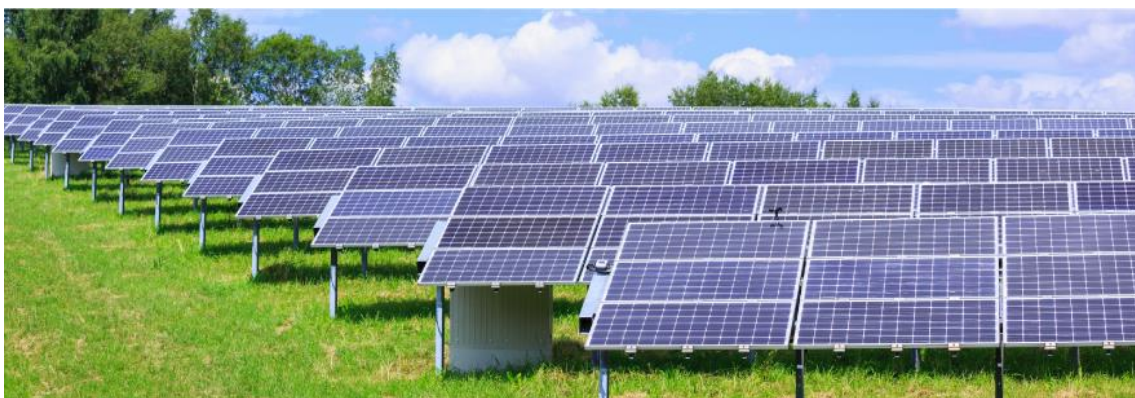
A solar farm
