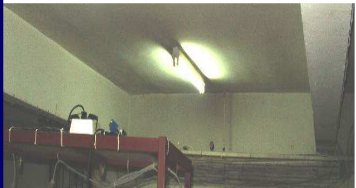
FIG. I.14. Photography of the buttresses (concrete beams) at the ceiling of the basement of Building B of the Faculty of Physics, measured with GPR on Figure 13.
