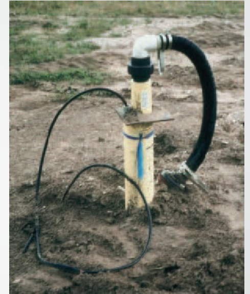
Recovery Well with Submersible Pump and Electrical Cord
