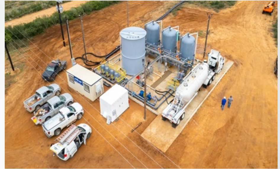
Satellite Resin Plant Maybe Built as Mobile Plant
