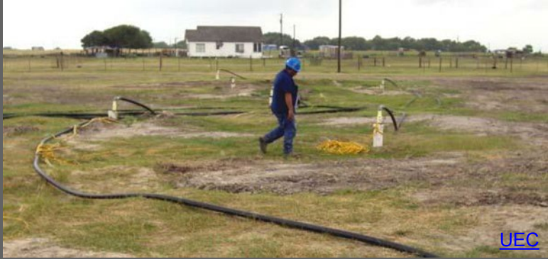
Typical Pattern Layout in Texas Production/Injection Piping on the Surface
